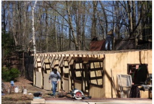
Six new enclosures take shape at Tom Ricardi's Birds of Prey Rehabilitation Center. Tom is in the forefront, Hobie Iselin and Brian Kuzmeskus, from left, work on the roof.
